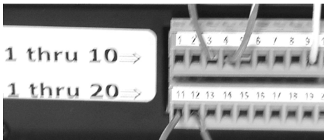
Figure 6. Black Wire to Terminal #12
